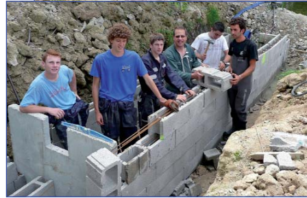
Our group had to overcome heavy constraints on a river-bed based construction site
